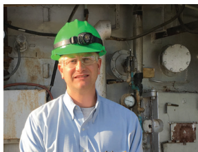
Kirk Oswald, utilities superintendent, stands in front of a combustion chamber of the Waste Heat Recovery Incinerator Unit he supervises.
