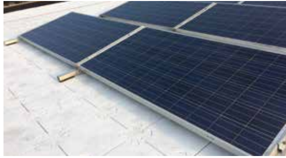
Solar panelling system installed on rooftop mounted with RoofClix panels.
